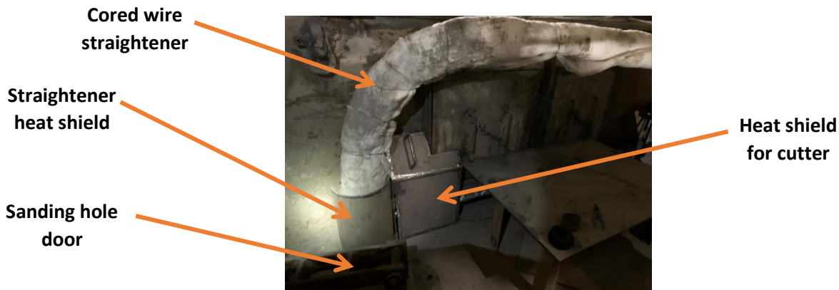
Figure 20: Installation of the cored wire cutter with the optical cored wire feeding system on the sump of the NSHC Consteel EAF.
