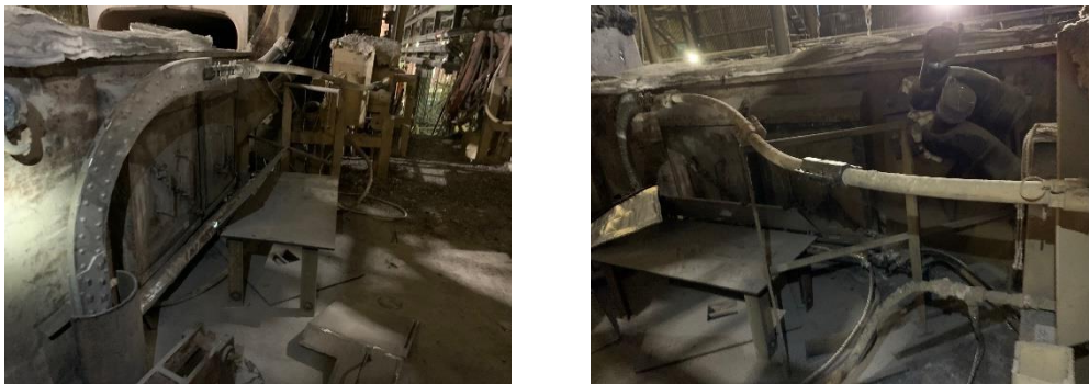
Figure 4. LEFT, picture of the CoreTemp installation on the EAF sump as viewed from the sanding hole. RIGHT, picture of the CoreTemp installation on the EAF sump as viewed from the wire feeder.
