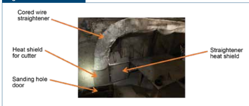
Installation of the cored wire cutter with the optical cored wire feeding system on the sump of the NSHC Consteel EAF.
